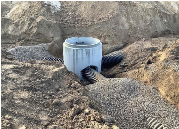
High School storm sewer system
