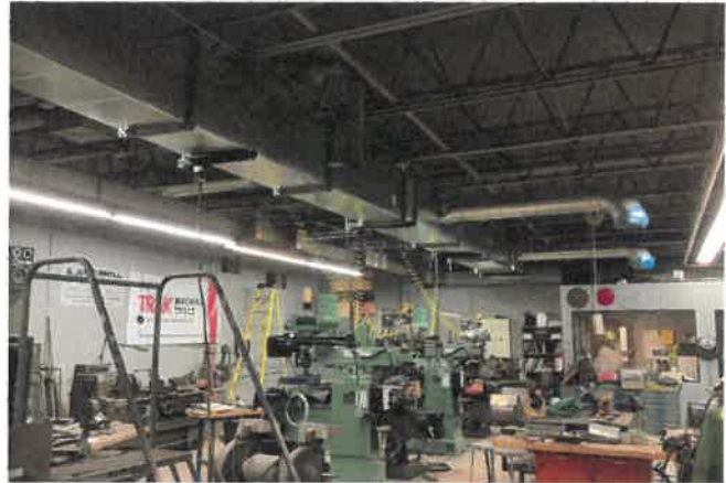
High School shop area mechanical installation
